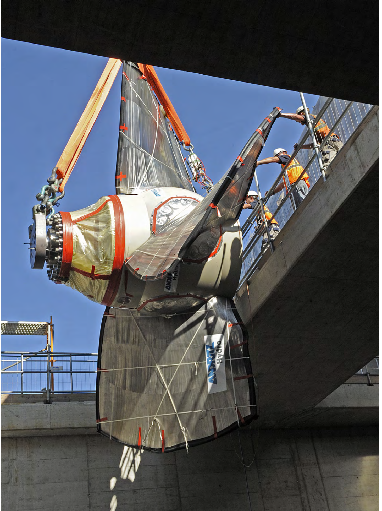
Images above and right Courtesy of Andritz Hydro
